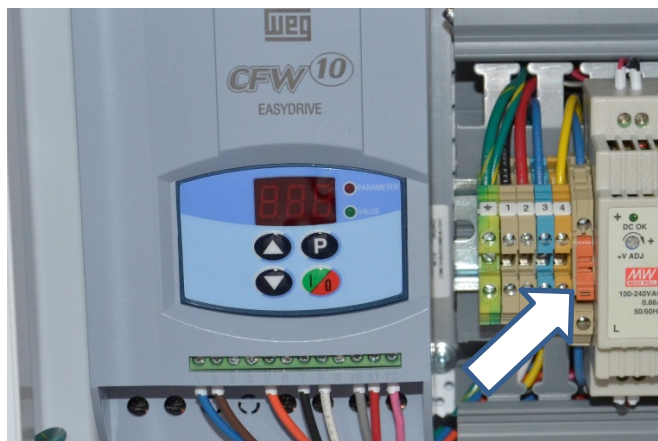
External Controls: Disable Manual Switch
